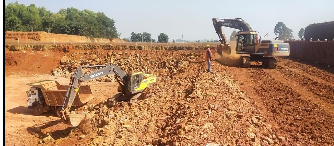
ROM & Primary Crushing
